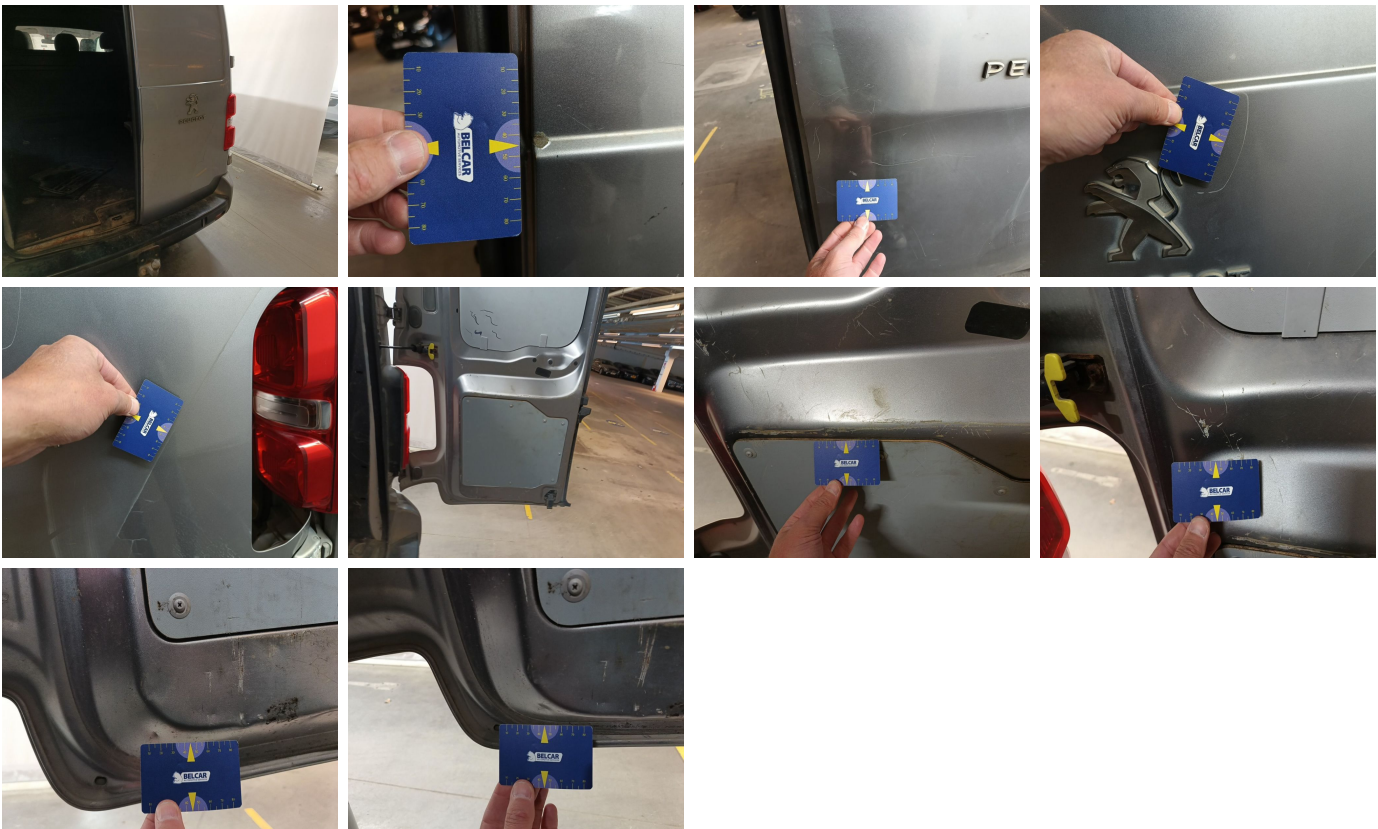
Rear Loading Door Right // Repair & Painting-scratch + dent
