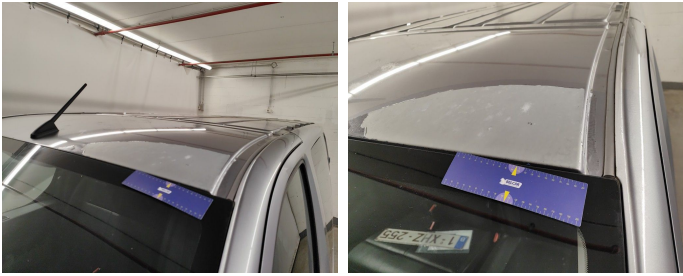
Roof // Painting-Chipped paint
