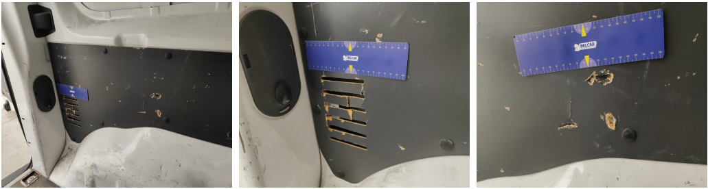
Interior // Repair 1-cracked
